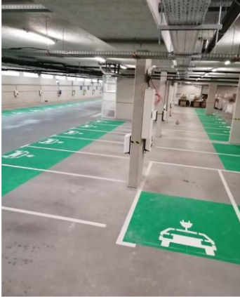
The charging plaza in Utrecht, launched in 2022, with 100 smart charging points
