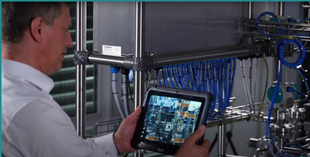
Figure 21 - How a maintenance worker can utilize augmented reality in the digital worker functionality to do their maintenance task.
